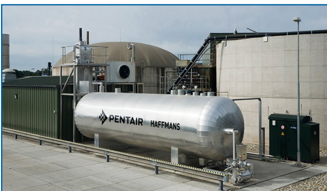
CO 2 Storage at the Ecofuels Biogas Upgrading Plant in Well, The Netherlands
