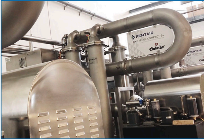
Pentair BMF System at Einbecker Brewery, Germany
