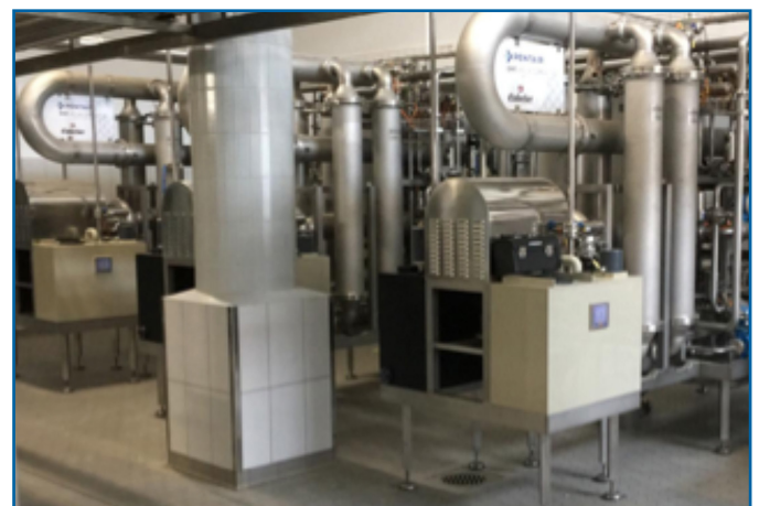
Pentair BMF System at Einbecker Brewery, Germany
