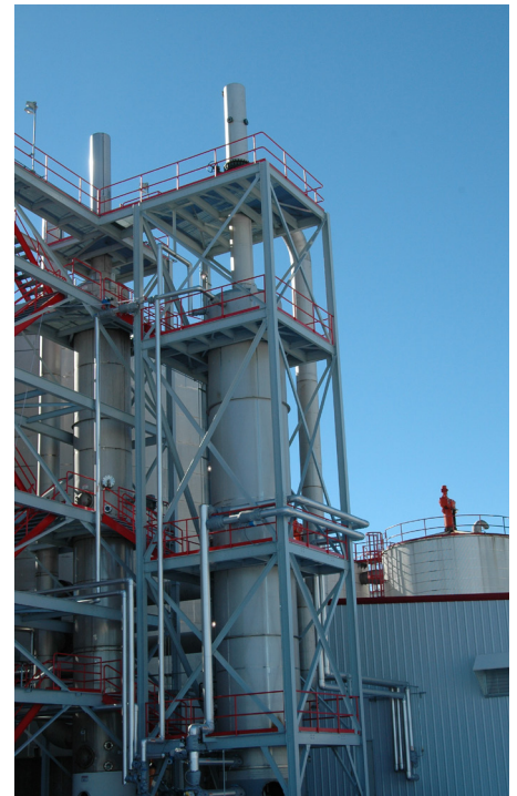
Ethanol Recovery System 2013
