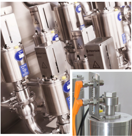
Shown above are process valves with proximity sensors equipped with finger protection guards. This solution for valve position feedback creates many challenges for plant operators.
